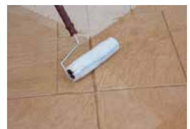
6. Aplicarea rasinii Sealfloor 100
